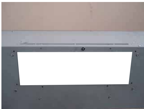
Horizontal Ducting (3-1/4"x10" Rectangular)
